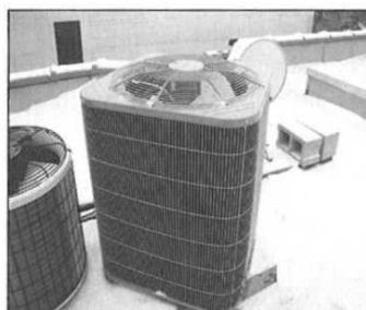
Air conditioning systems
