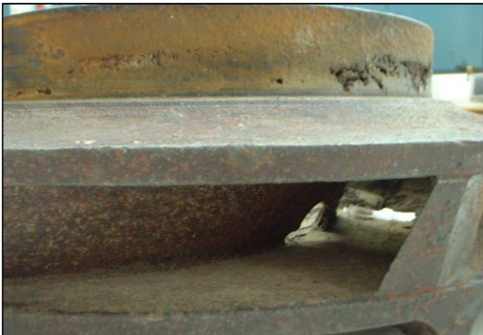
Figure 1.25. Consequence of cavitation damage on an impeller of a pump. Profile view
