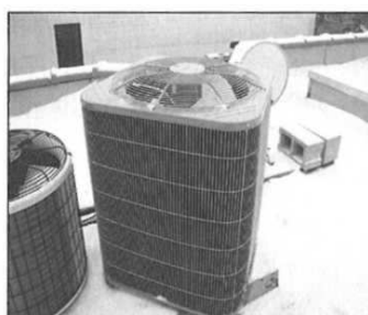
Air conditioning systems
